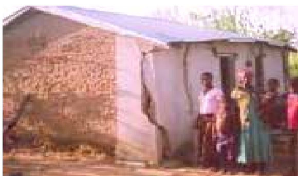
Photo 2: Damaged rural housing in Aklakou
