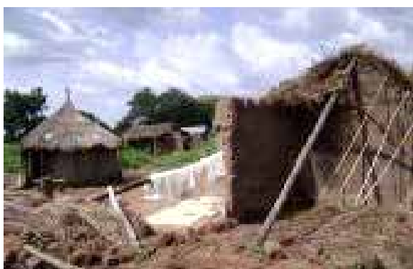
Photo 3: Mud and straw huts destroyed in Tokpli
