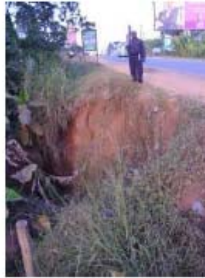
Soil erosion from uncontrolled stormwater run-off
