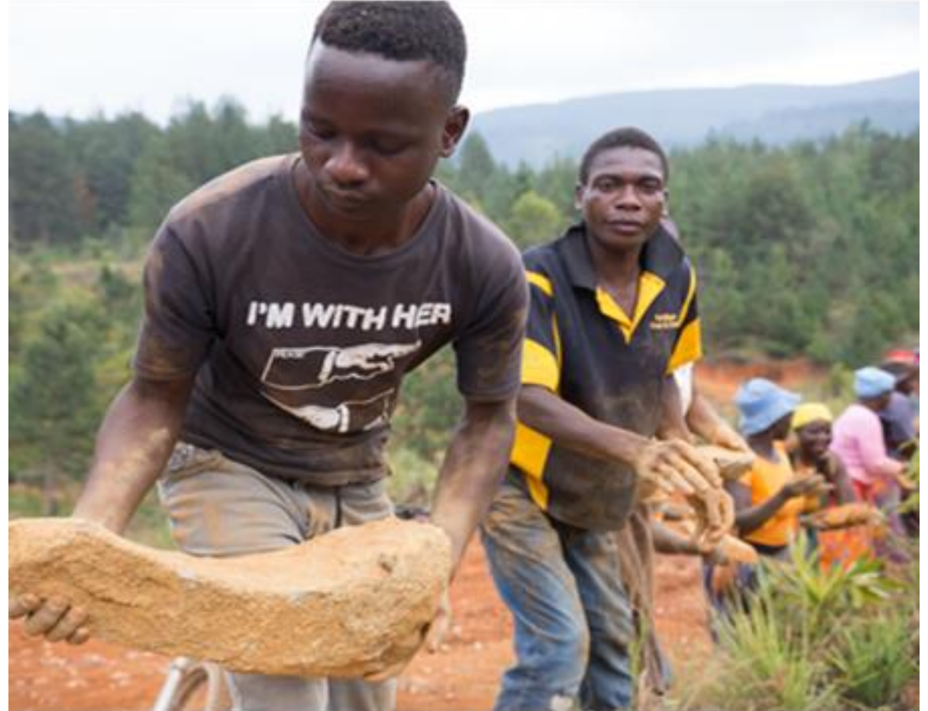
Community rebuilding their dip tank using BBB principle in Ward 22 of Chimanimani District.
