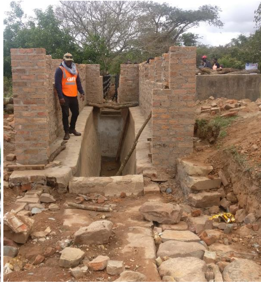
Rehabilitation work at Chikore dip tank, in Chipinge, is at final stage.
