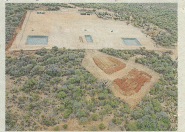
A coal plant construction site in Lamu in a picture taken February 1, 2018. Picture: File
